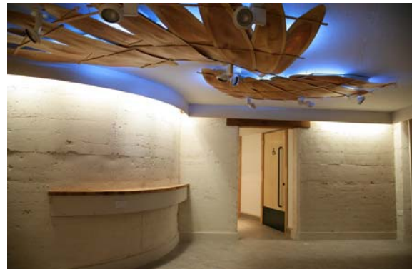
The pelmet above conceals cables as well as provides the perfect mounting location for wall washing
